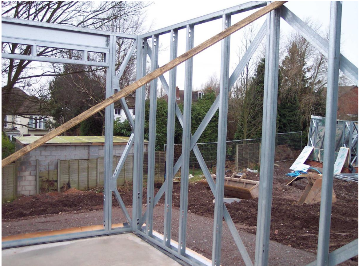
FIGURE 22 - STEEL FRAMES. C SECTIONED STEEL STUDS WITH FLAT DIAGONAL STRAPPING ON OUTER SURFACE
